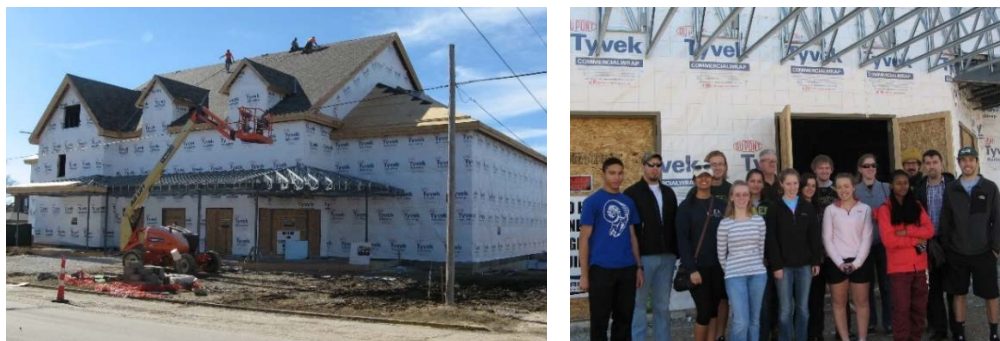
Figure 3. Visiting of Missouri S&T Phi Kappa Theta Fraternity House construction site in Rolla, Missouri in spring 2015 semester
