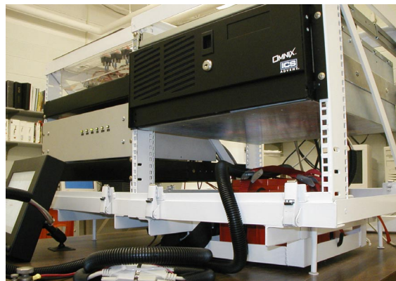
Fig. 9. Electronic rack assemblies.
