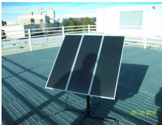
Figure 16. solar panels used to power hydrolysis system
